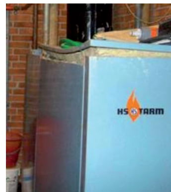
Hyllehøjskole – 22 year old boiler at school – to be upgraded
