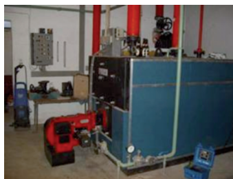
Hyllehøjhallen – 24 year old boiler at sport facility – to be upgraded
